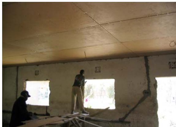
Renovating classroom at Ilkiding'a Secondary School to house 30+ desktop computers, printers, and scanners; bringing countless new resources to the village.
