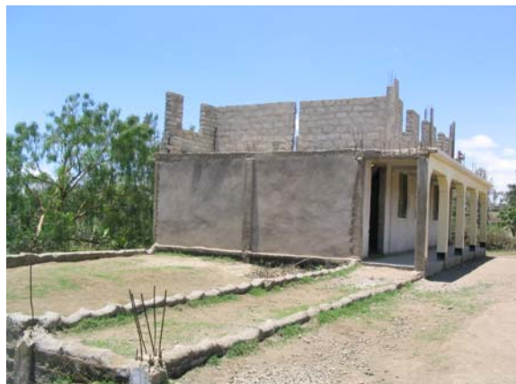
Classroom construction at Natema Primary School. Funds are needed to complete the upstairs classroom.
